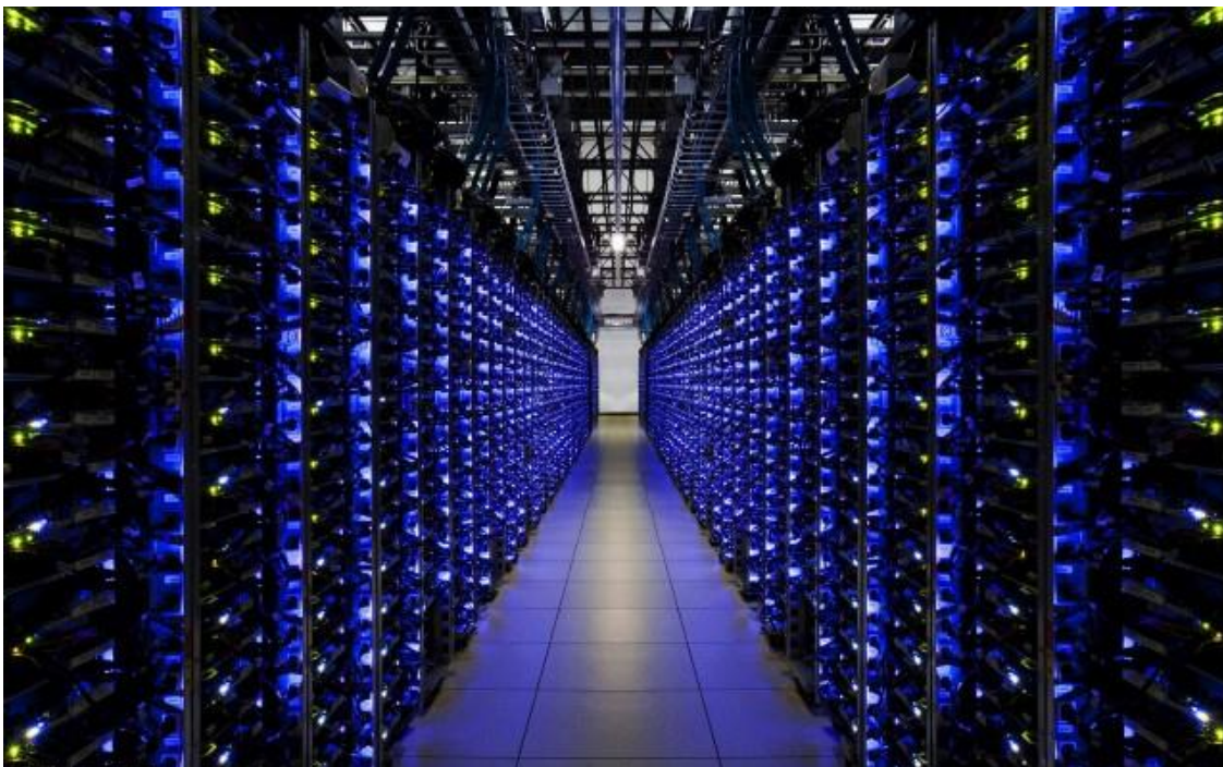
A typical Data Centre
